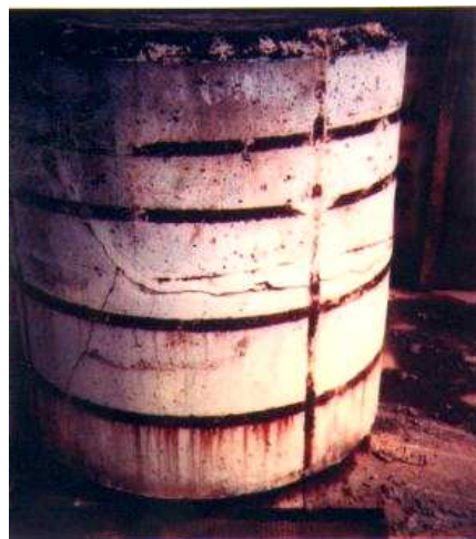
Fissured concreted hull
